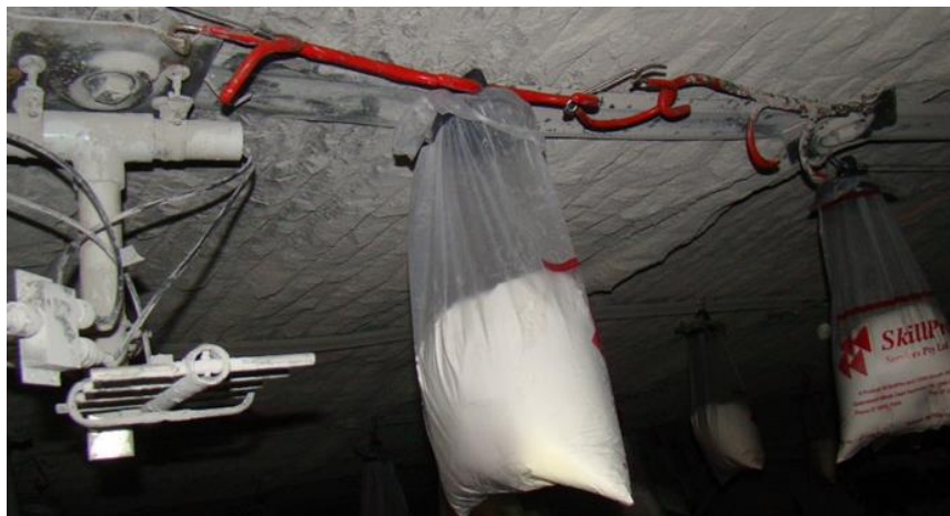
Figure 4.5: Rubber Coated Cable Hanger Support Method
