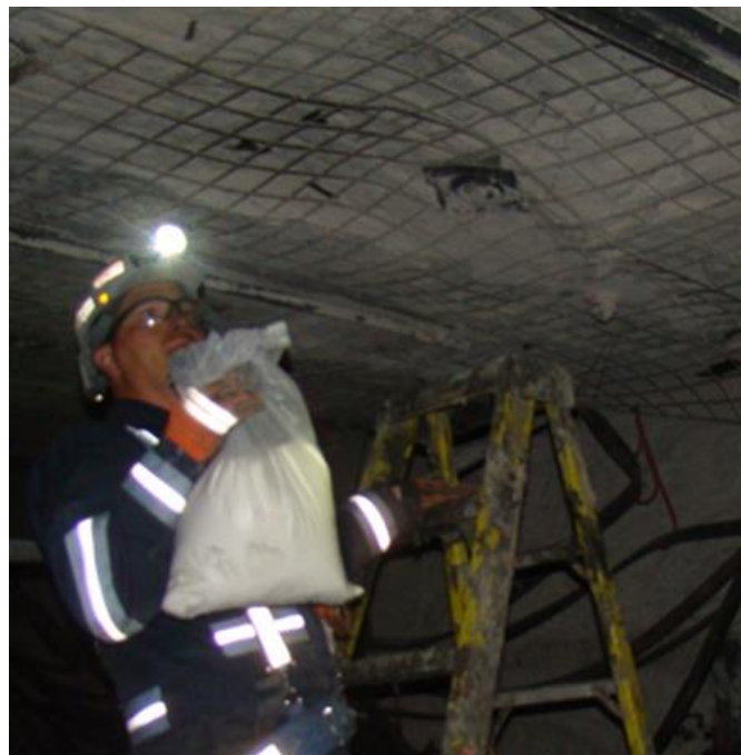
Figure 4.8: Miner Hanging Bag from 8 Foot Ladder
