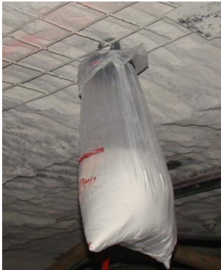
Figure 4.9: Barrier Bag Hung from Roof Mesh
